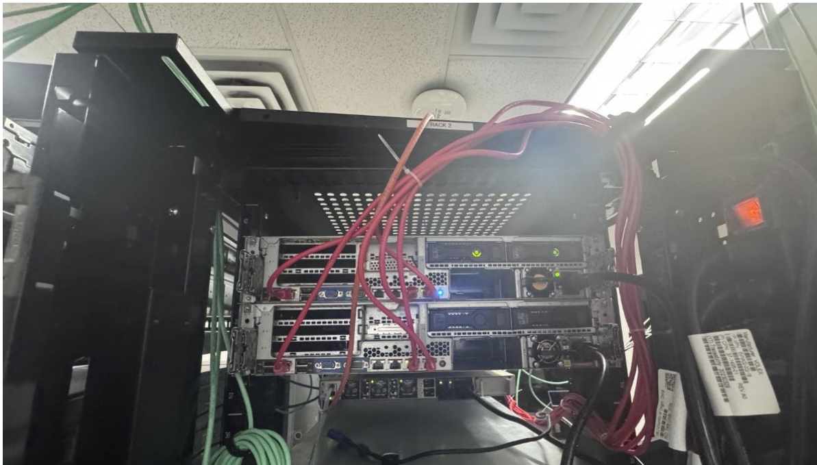
Figure 4. Site 1 rack installation (rear view)
